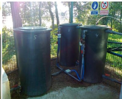
Tanks for reclaimed water and one with \text{CO}_2 injection (right tank).
