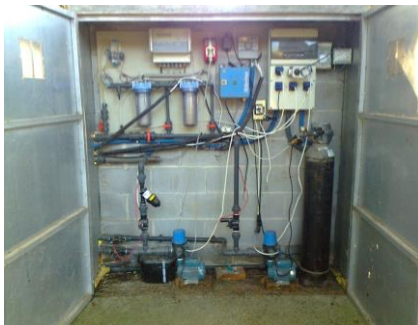
Automatic control panel for irrigation schedule and \text{CO}_2 injection
